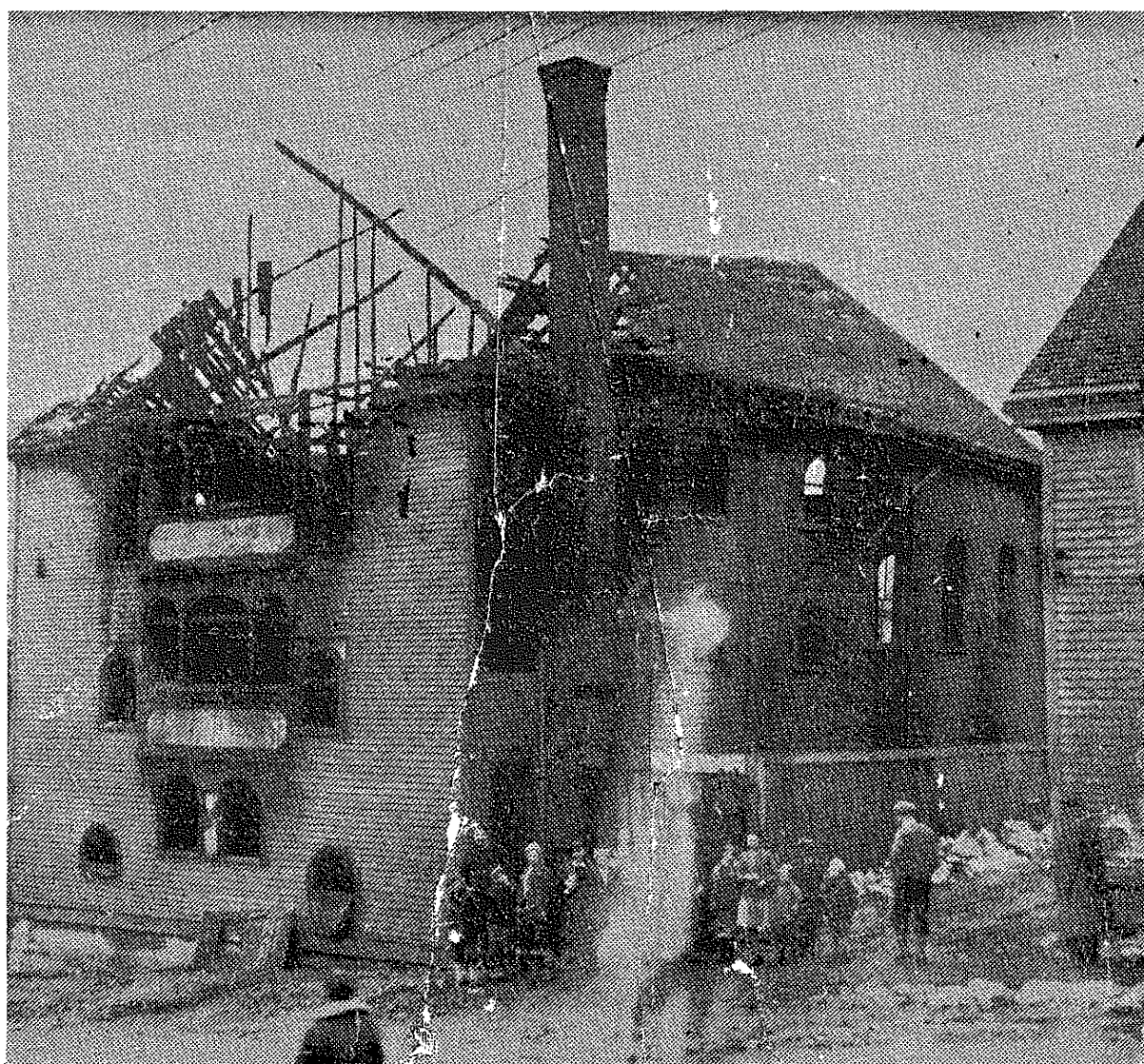
BETH ABRAHAM SYNAGOGUE Aftermath of the disastrous fire on Carr Street, March 30, 1932.
